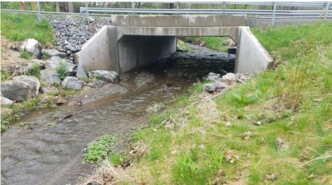
Ancram, with NY State aid, was able to enlarge two culverts to prepare for flooding events. Photo courtesy of Colleen Lutz.
